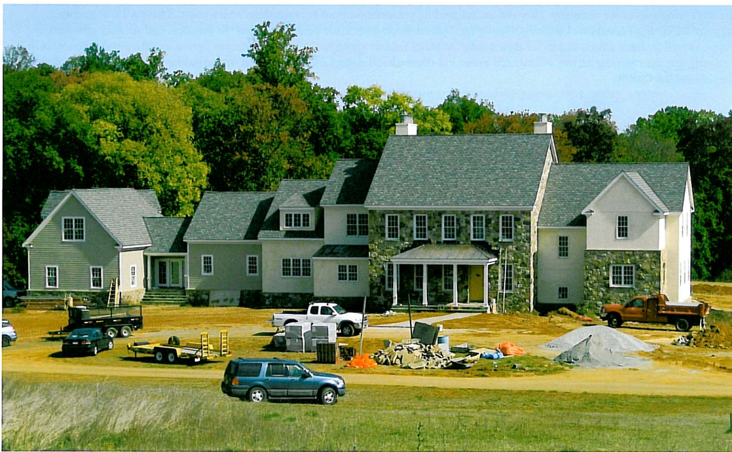
Foster-Herz, Inc. is building this beautiful 14,000 sq. ft. custom home on 25 acres in south Leesburg, VA. It will have 3 furnished levels with 4 bedrooms, 8 baths and a complete in-law suite above the garage.
